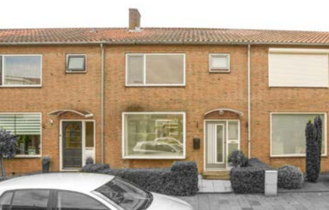
ponsgaten in metselwerk, rode pan, repeterende woning, vlakke gevel
